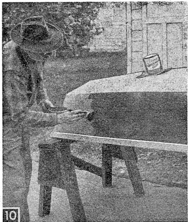
Apply generous coating of Elmer's Waterproof Glue to bare plywood in preparation for muslin covering. Stretch muslin tightly over glue, then squeegee flat. When glue is set, but not rock-hard, trim edges with razor blade. Around corners, cut out muslin to prevent overlap as ends are wrapped over edge.
